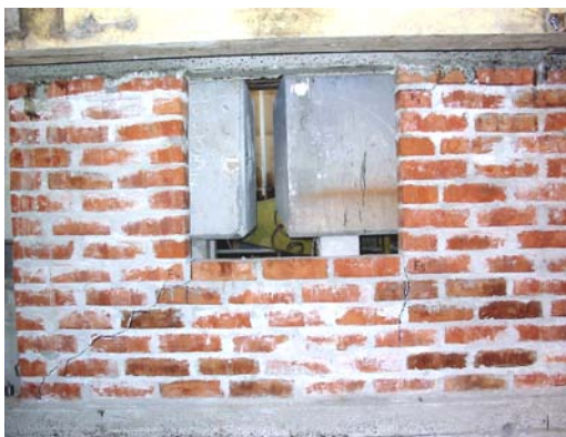
Failure pattern of masonry wall
