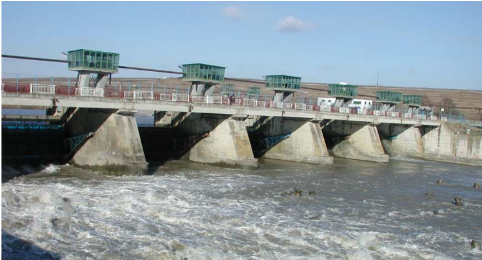
Figure 1 Dam river on Mures River at Mintia
